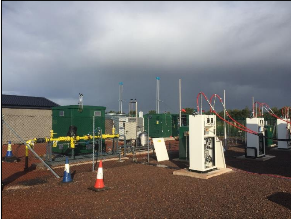
Meter, Odorant Unit, CV Measurement and Dispensers
